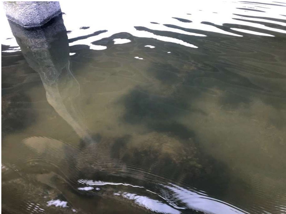
Figure 4.3. Tubeworms are also present in clumps beside the bridge piles.
